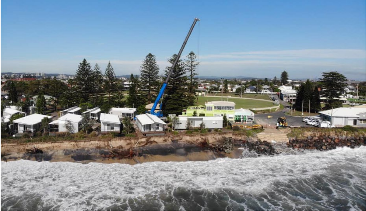
Cabins being removed from the caravan park due to beach erosion following a large wave event in February 2020.
