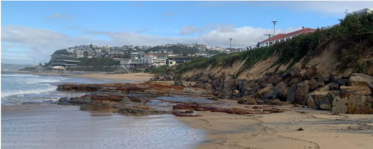
Figure 4: Pogos rock platform and exposed lower slope rock armour in John Parade revetment following storms in 2021.
